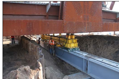
Figure 7 - Push/Pull frame and reaction sled used for horizontal sliding of trusses shown at job site
