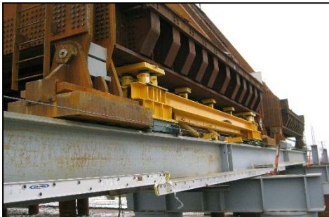
Figure 6 - Push/Pull frame and reaction sled used for horizontal sliding of trusses shown at offline location
