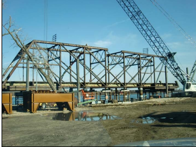
Figure 12 - Existing approach span truss with portion of top chord and diagonal removed
