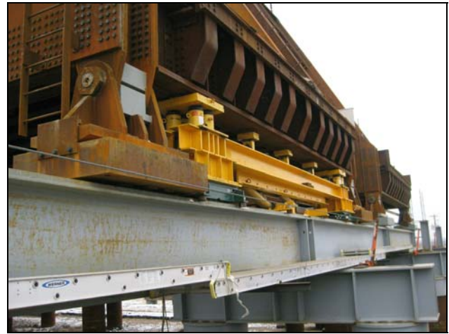
Figure 6 – Push/Pull frame and reaction sled used for horizontal sliding of trusses shown at “Green Bay” location
