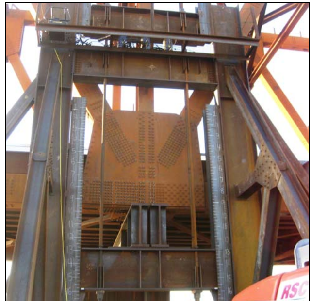
Figure 11 – Side view of jacking tower and “lifting beam” used for truss float-in
