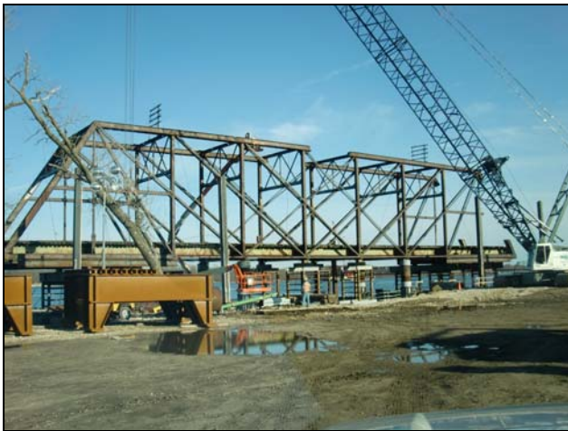
Figure 20 – Existing approach span truss with portion of top chord and diagonal removed
