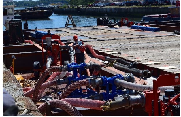
Figure 16 - 6" Ballast Pumps (16 used)
