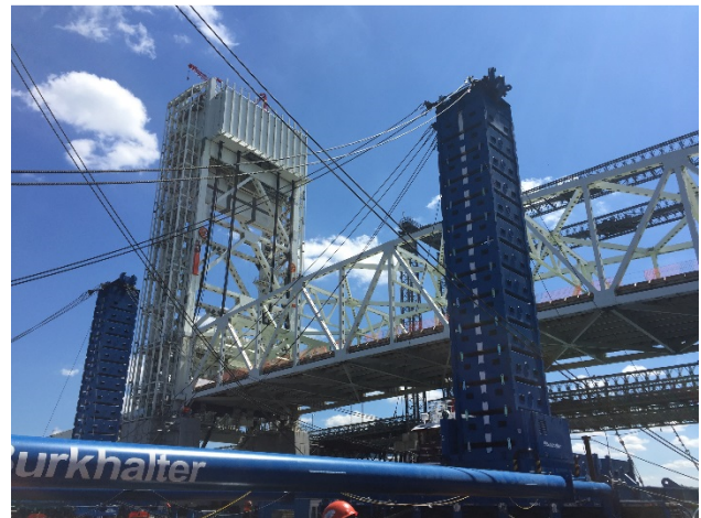
Figure 26 - Sagging Main & Tower Stability Lashing
