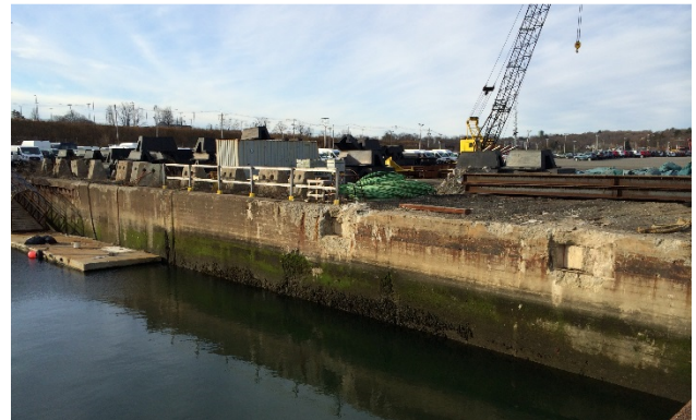
Figure 13 - Wet Basin Wall (Ramp landing Area)
