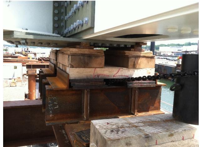
Figure 9 - Bearing Bar Location had Tight Tolerances
