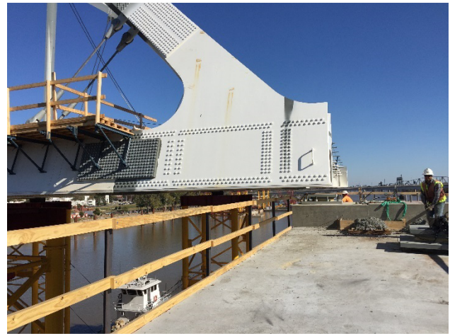
Figure 20 - Knuckle Clearance above Bearing
