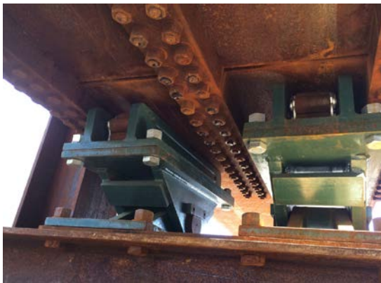
Figure 7 – Launch Rollers & Splice Interface
