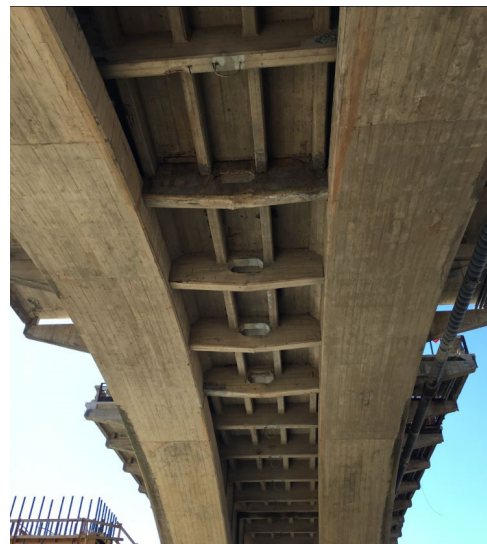
Figure 7 – Large Holes in Capbeams
