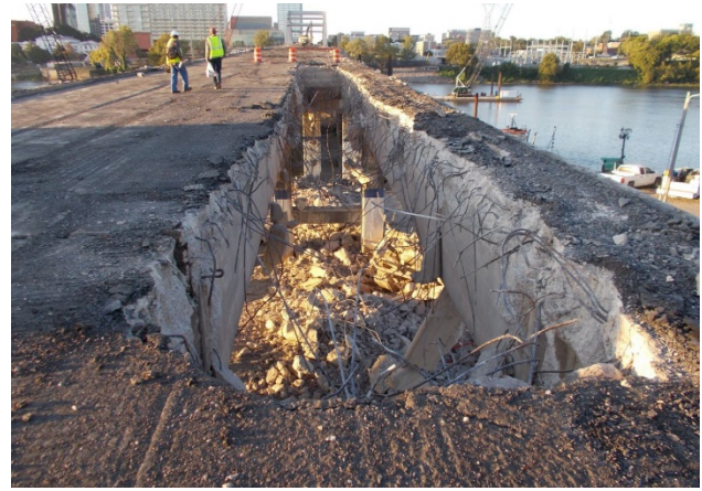
Figure 13 – Deck Removed Between Girders
