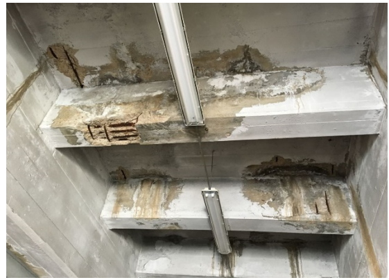
Figure 4 – Exposed Reinforcement in Beam
