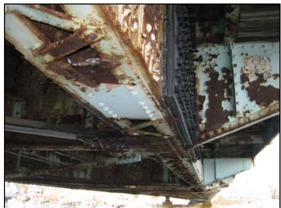
Figure 3 – Deterioration of lower chord and floor system After extensive research and community outreach,
