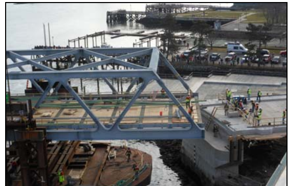
Figure 25 – South Fixed Span Truss rotated into position to set down on permanent bearings
