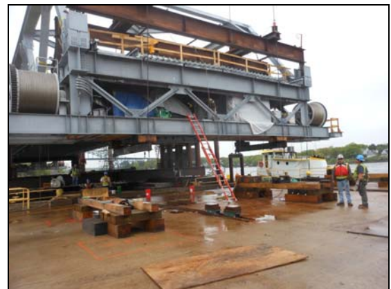
Figure 22 – Machine Room fully installed
