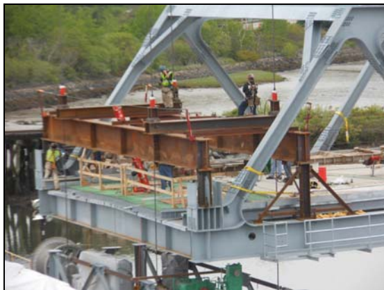
Figure 20 – Jacking Grillage for machine room lift, grillage supported by bottom chord of New Lift Span Truss
